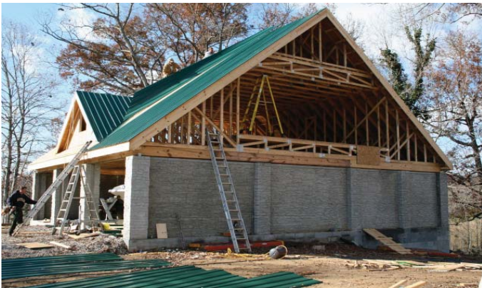
Above: Pour in Place using the versatility of the Verti-Crete System to build a garage suitable for a motor home.
