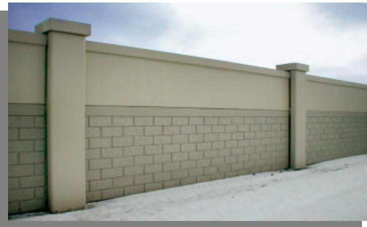
The new concrete installation is impervious to UV damage, can withstand the heavy winter salting of Minnesota roads, and is less likely to sustain serious damage from road traffic
