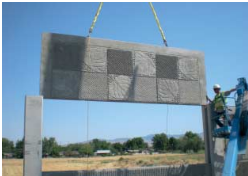
Fig. 1 The wall side facing the freeway got a leaf and fractured fin design.
